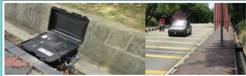
Figure 2: RealCount™ ATC installed on the road
